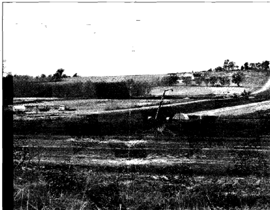
HEAVY-DUTY WORK: Construction on the dam that will form Lake Wanhoo began this fall just north of Wahoo.
