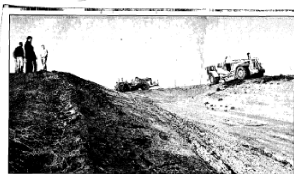
UNDER CONSTRUCTION - While groundbreaking participants watch, dirt movers from Commercial Contractors of Lincoln pull soil from the top of Bodley Hill down into the Sand Creek valley were the Lake Wahoo dam will sit.
